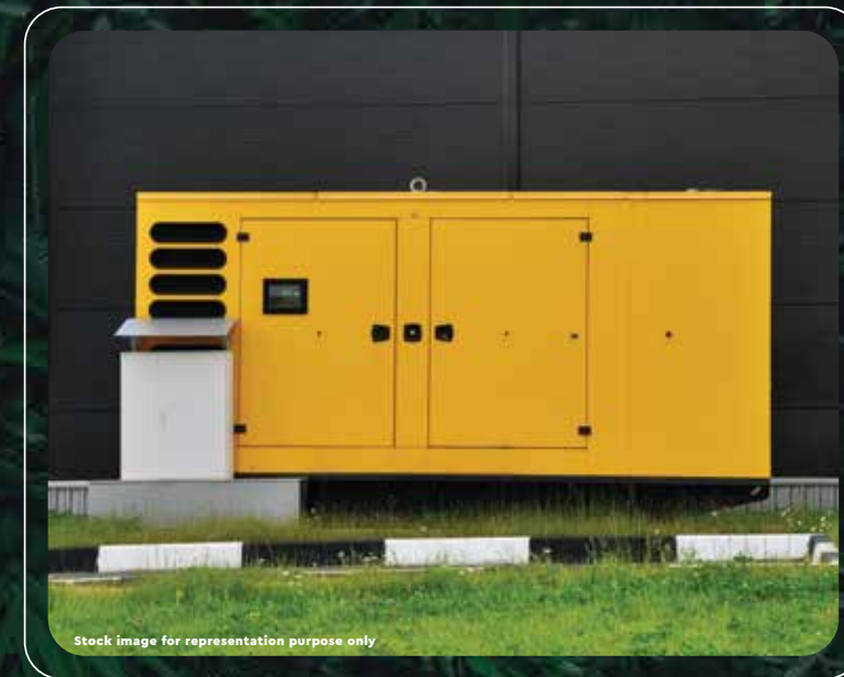
Power backup in common areas
